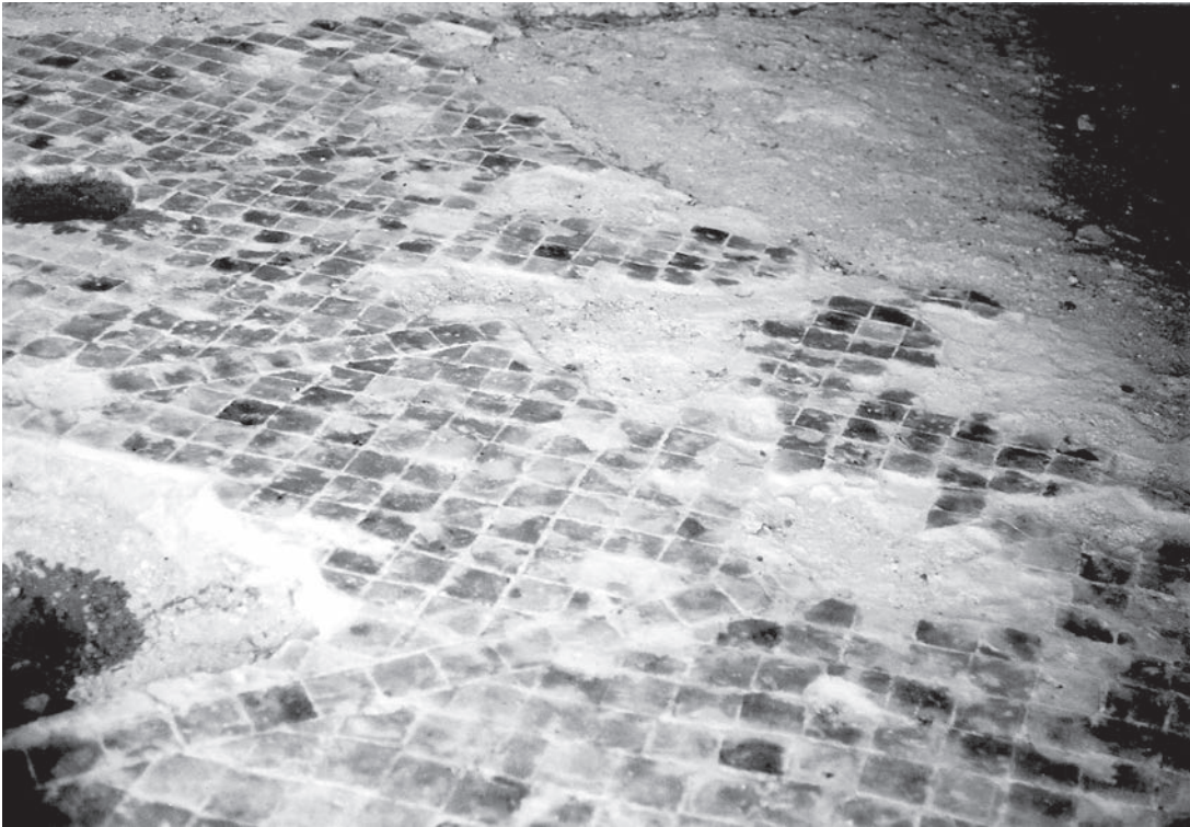
Figure 1.2 Part of the thirteenth-century refectory floor at Denny Abbey, Cambridgeshire, showing the diagonal format with single lines of tiles inserted.
